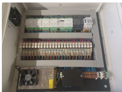
Upgraded module for the DC system.
