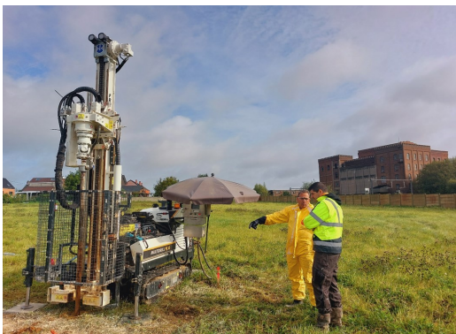
Injection equipment at the NAM site.
