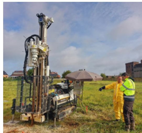
Implementing monitored bioaugmentation technology at a site in Belgium. Injection rig for adding oxygen to ground is shown
