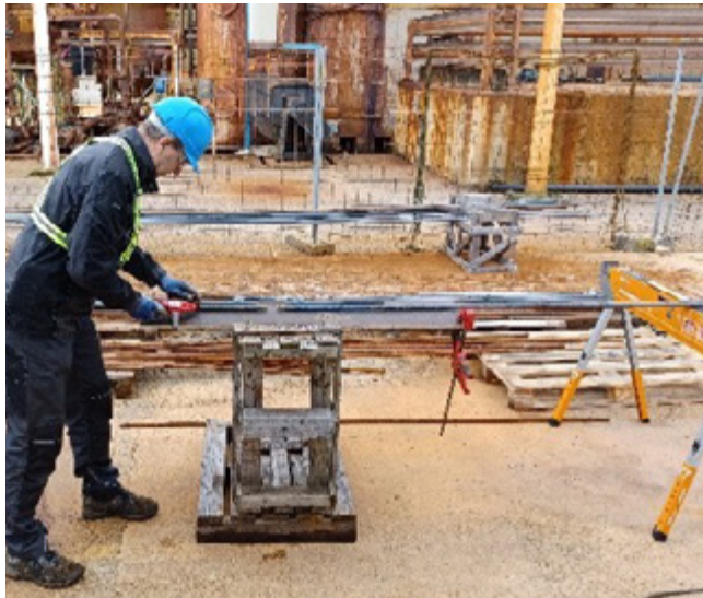
Preparation of a new set of power electrodes for regular replacement
