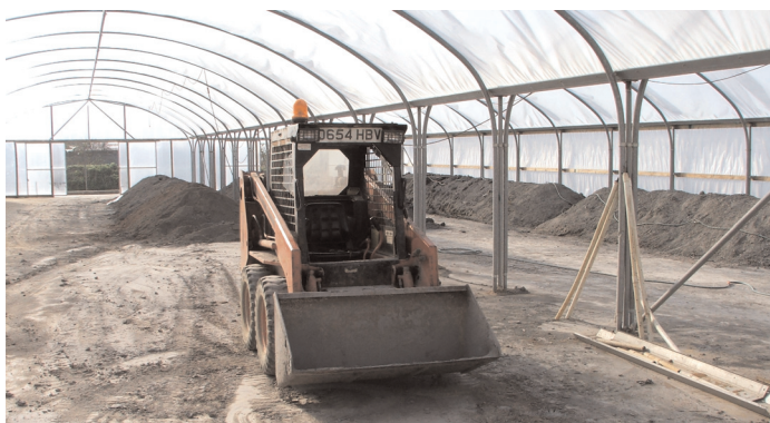
Figure 1: Biopile treatment unit of the field trial carried out during PROMISE project (©Remedios Ltd).
