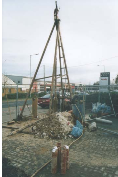
Plate 4.2: Collection of rock core samples from the unsaturated zone in the site source area using percussion drilling methods. Core samples are shown in the foreground.
