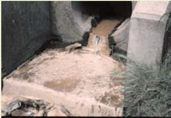
Figure 5: Quaking Houses - Pollution of the Stanley Burn with iron and aluminium oxyhydroxides.
