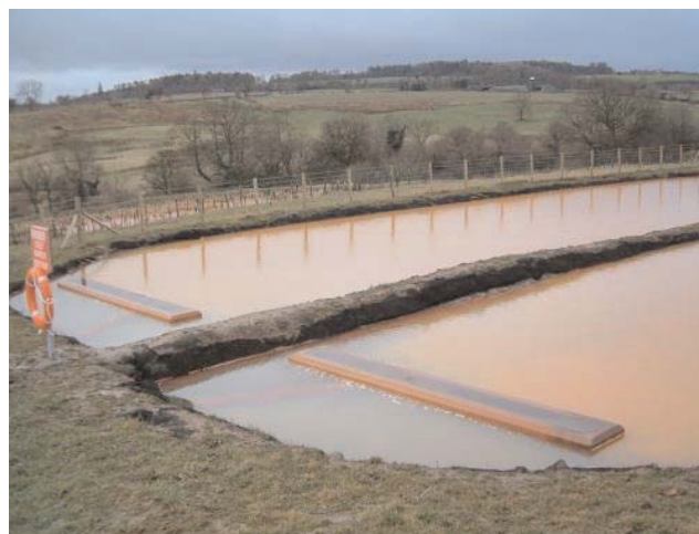
Figure 10: Whittle - parallel settling ponds.
