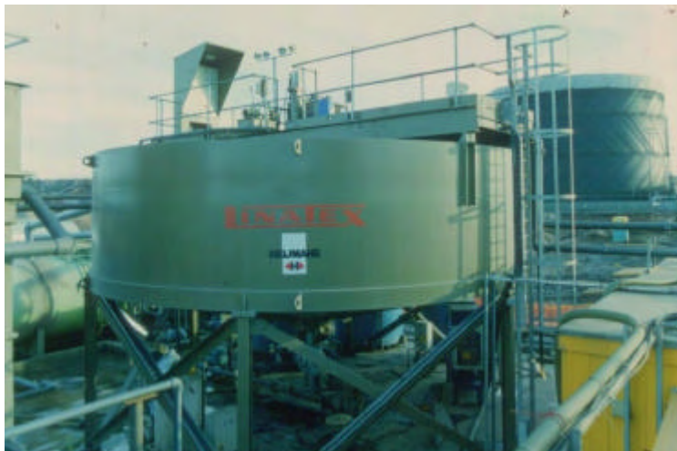
Plate 6: Water treatment system.
