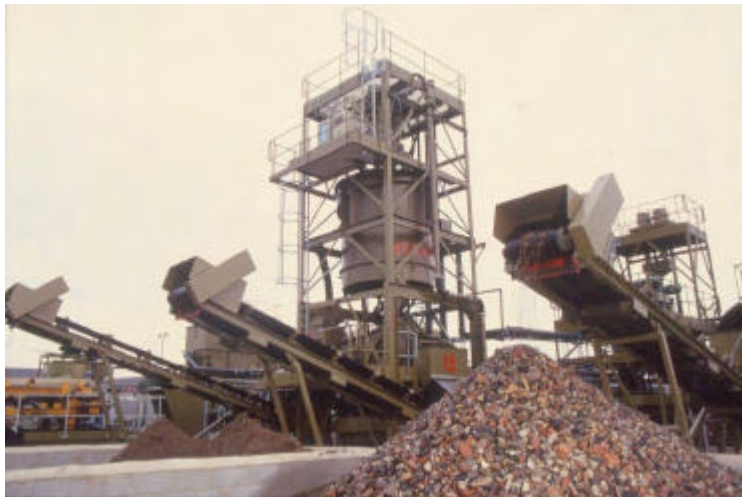
Plate 2: Clean coarse output from soil washing plant containing natural and made ground.
