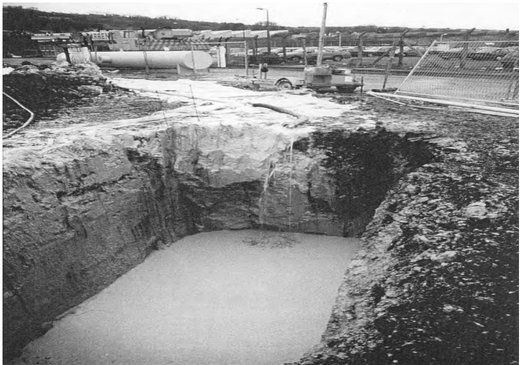
Plate 6.3: Wall enlargement for reaction vessel. Reaction vessel in the background. Source: Golder Associates (1996)
