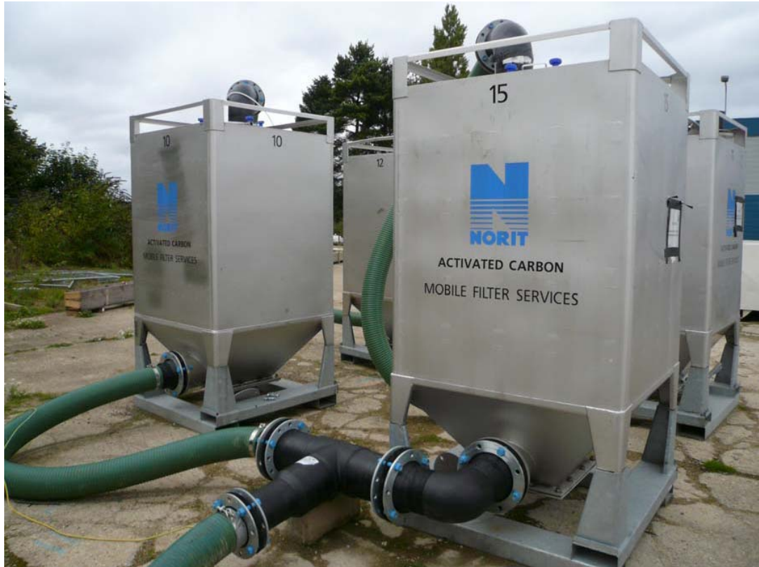
Plate 6.3: GAC off-gas treatment system
