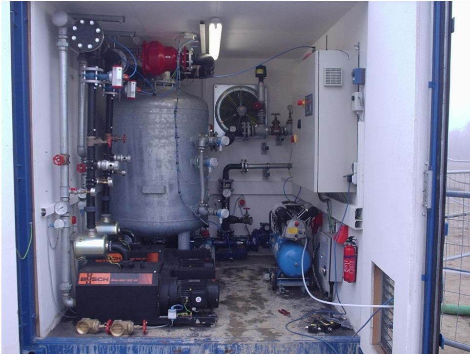
Plate 5.2: Pilot trial SVE plant
