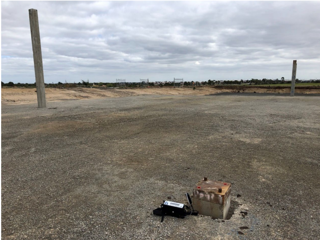
Figure A2.14: Gas monitoring around the top of driven precast concrete piles
