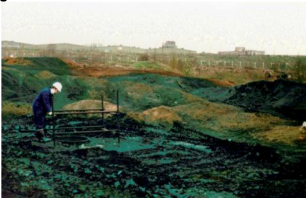
Photograph 37. Spent oxide. Source: Russell Thomas.
