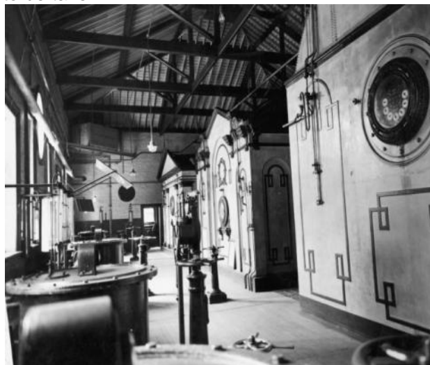
Photograph 42. Station meters (right) in the meter house.
