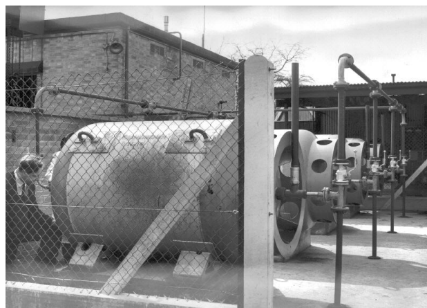
Photograph 51. A small butane air plant.
