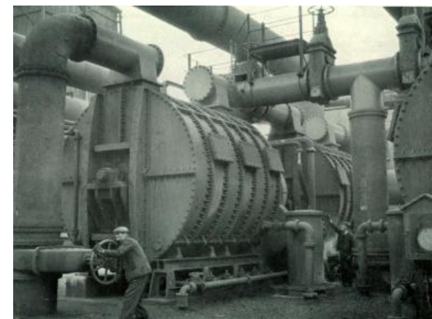
Photograph 48. WC Holmes dri-gas plant at the former Beckton gasworks.
