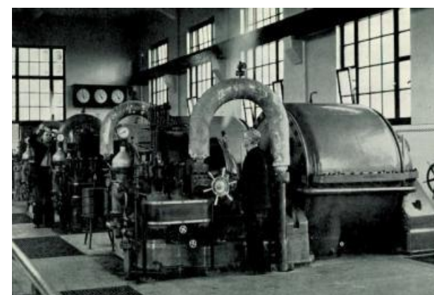
Photograph 52. Four high-pressure turbine-driven boosters at the former Beckton gasworks.
