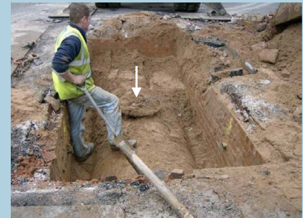
FIGURE 16 Pipe lifting point identified
