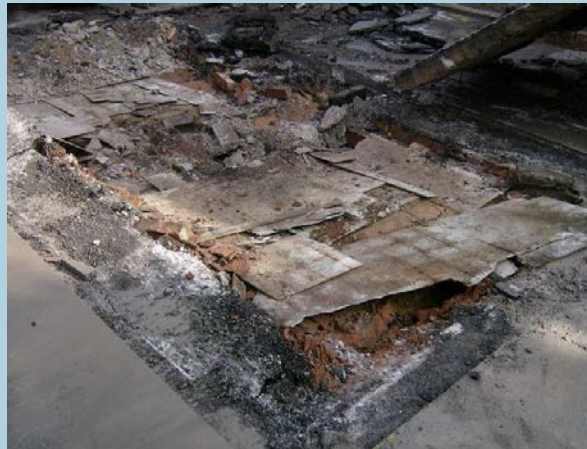
FIGURE 14 Asbestos sheeting found
