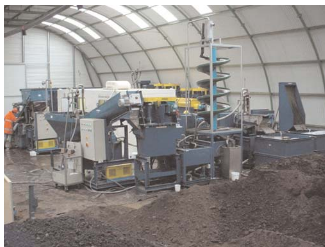
Figure 1: General layout of the soil washing plant.
