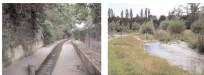
Figure 11. Process of repositioning a concrete lined channel into a new riverbed at Chinbrook Meadows (Greater London, UK), showing original concrete lined channel (left) and new channel floodplain protection (right). Picture courtesy of the River Restoration Centre (RRC).
